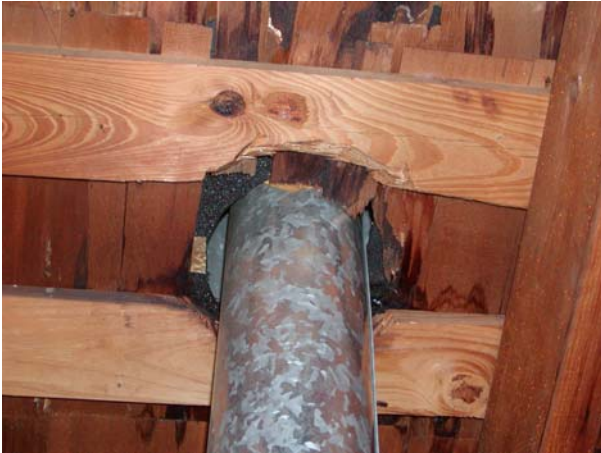
Furnace vent pipe in contact with wood roof
